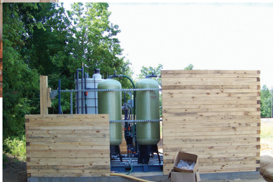
Small groundwater treatment system with two tanks of GAC.
