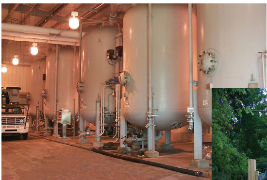
Large groundwater treatment system with five tanks of GAC.
