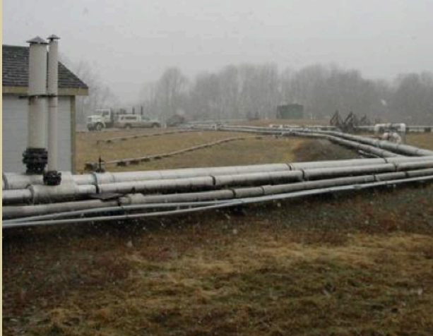
Bioventing system at drum disposal area, DS&G Landfill
