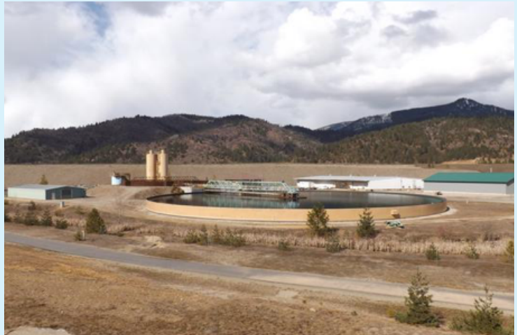
EPA-operated Central Treatment Plant, where EPA is currently treating the acid mine drainage coming from the Bunker Hill Mine
