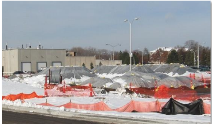
Figure 3. Covered piles of excavated soil during cleanup of the Cummins ATC area. Image source: MPCA
