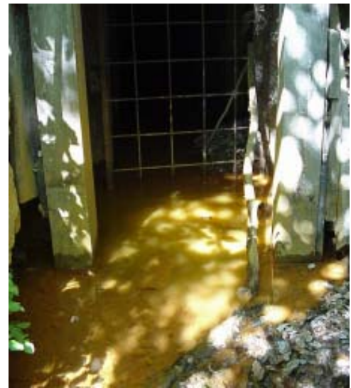
Acid mine drainage leaking from the Stowell portal at Mammoth Mine, California.
