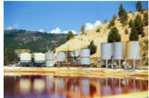
Bi-phasic chemical treatment system of acid mine drainage at Leviathan Mine, California.
