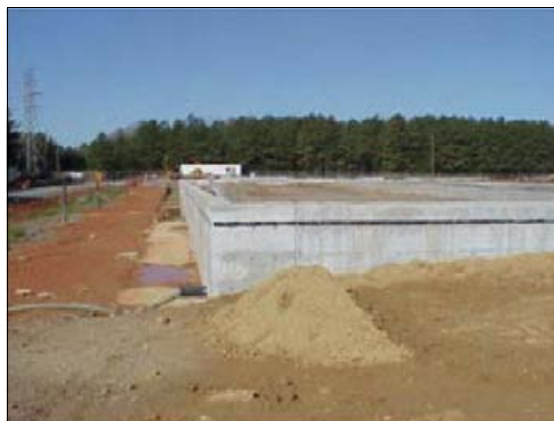
Construction of “divider wall” at the Rentokil site. All development must occur within the walls to prevent cover disruption.
