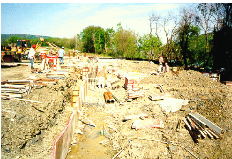
Construction of a slurry wall at the Ohio River Park Superfund site in Neville Island, Pennsylvania.
