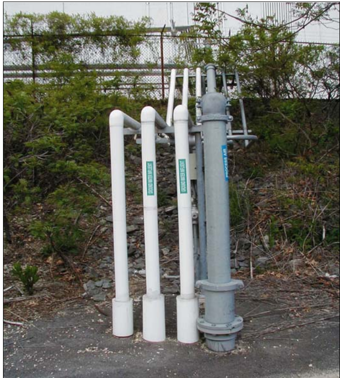
Piping for groundwater treatment at the Peterson/Puritan Superfund site in Cumberland and Lincoln, Rhode Island.
