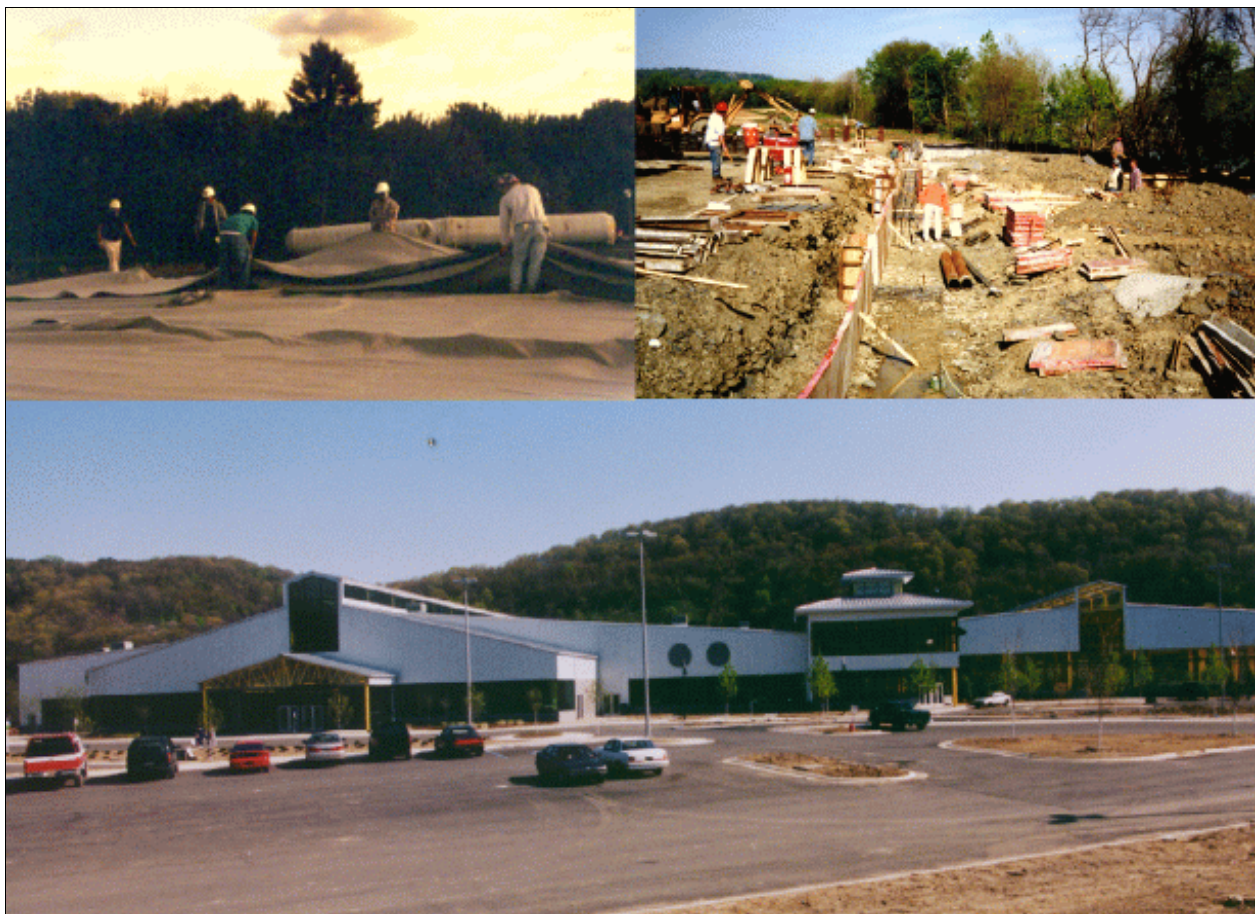
Protective cover installation, slurry wall construction, and the completed Island Sports Center.
