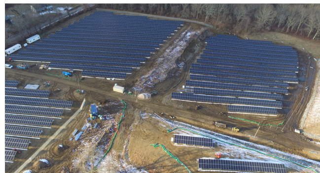
Figure 136. Drone image of the solar farm installed at the West Kingston Town Dump/URI Disposal Area site (Rhode Island). Photo used with permission of Kearsarge Energy.
