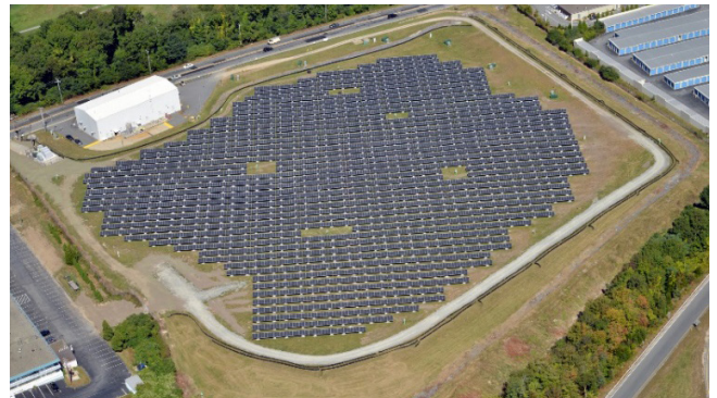
Figure 96. Aerial view of the solar array at the Sullivan's Ledge site (Massachusetts).
