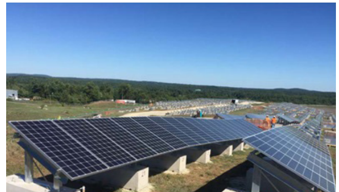
Figure 77. Solar panels at the Charles George Reclamation Trust Landfill site (Massachusetts).
