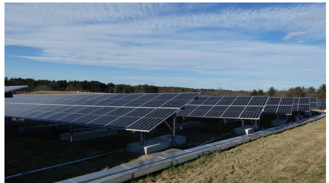
Figure 97. Solar panels at the Sutton Brook Disposal Area site (Massachusetts).
