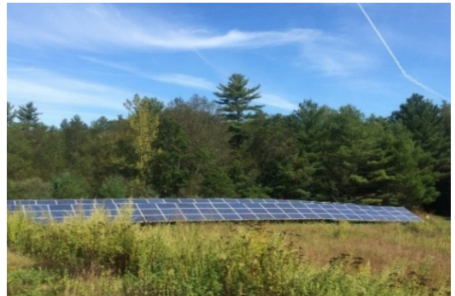
Figure 92. Solar panels are used to power the groundwater treatment system at the Re-Solve, Inc. site (Massachusetts).
