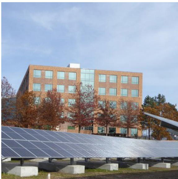
Figures 26 & 27. New solar arrays at the Industri- Plex Superfund site (Massachusetts).
