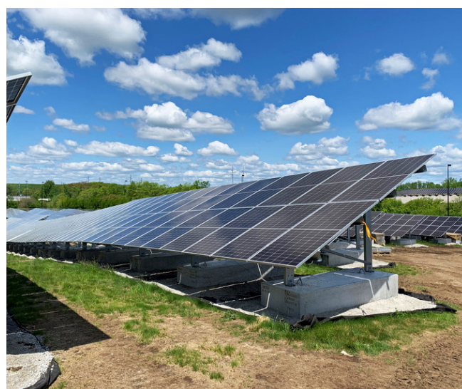
Figure 84. The new solar array at the Industri-Plex site (Massachusetts).
