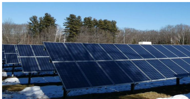
Figure 80. The solar facility at the Groveland Wells site (Massachusetts).
