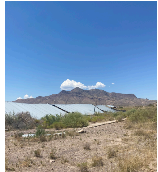
Figure 1. Collapsed buildings at the Eagle Picher Site.
