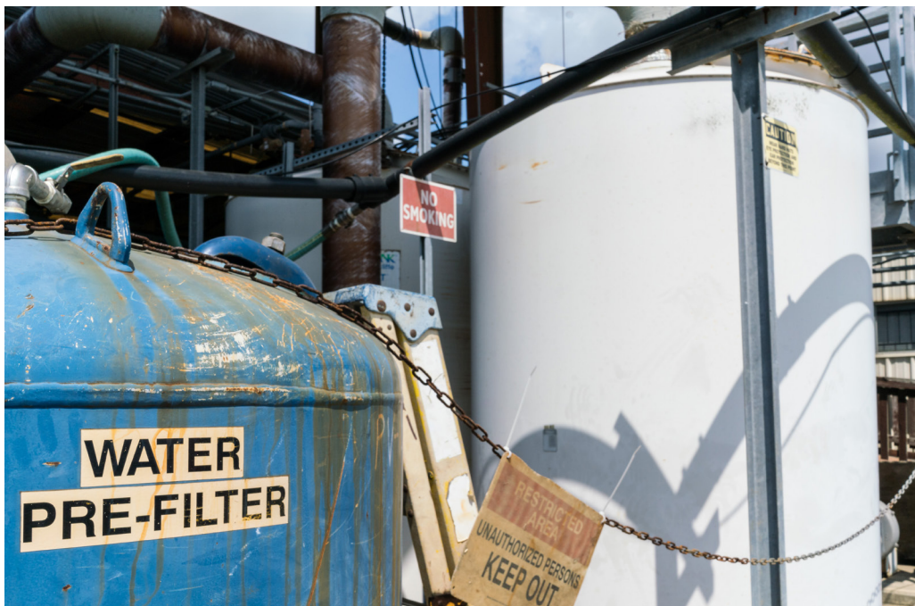
Figure 16. A separator system to remove contaminants from groundwater.
