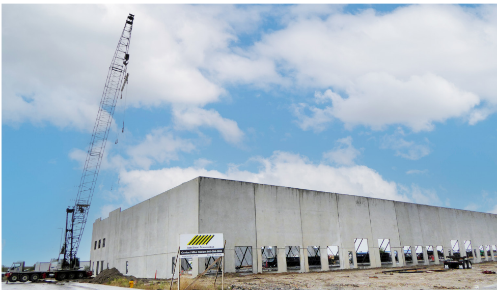
Figure 18. The Redwood Depot warehouse project underway at the Portland Cement (Kiln Dust 2 & 3) Superfund site (Utah).
