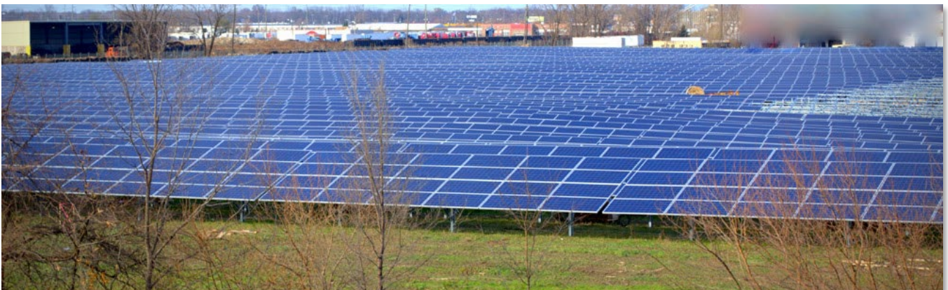
Figure 4. View of Maywood Solar Farm at the site.
