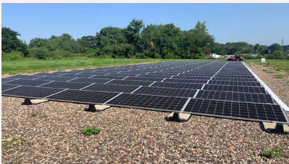
Solar photovoltaic (PV) panels
