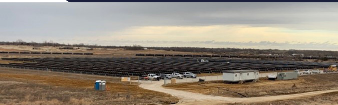
Figure 4. The 12-acre, 2-megawatt community solar farm pilot on site
