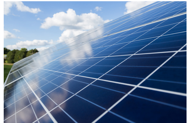
Figure 19. A solar array will power to the groundwater treatment system at the Allied Chemical & Ironton Coke site (Ohio).
