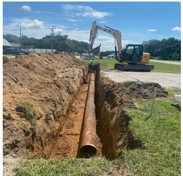
Figure 15. At the Arkla Terra Property site, cleanup included connecting affected properties to the public water supply (Florida).
