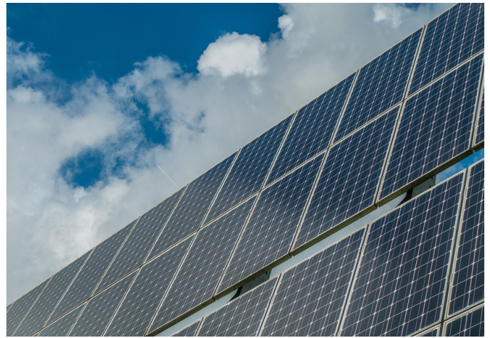
Figure 20: Solar power generated at the Combe Fill North Landfill site (New Jersey) will help the state achieve its clean energy goals.
