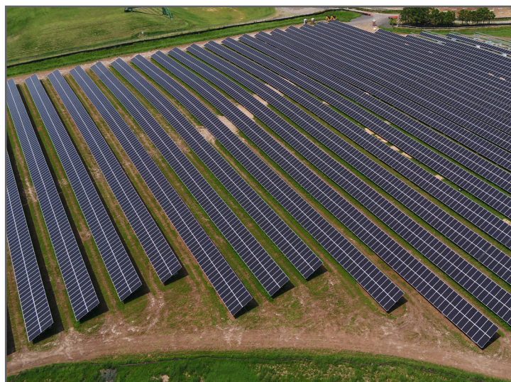
Solar array at the Ciba-Geigy Corp. Superfund site in Toms River, New Jersey.
