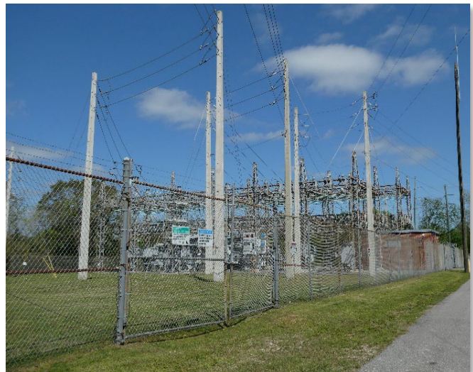
Figure 32. The JEA substation.
