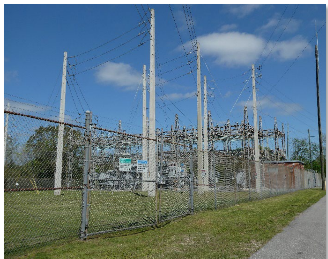
Figure 32. The JEA substation.
