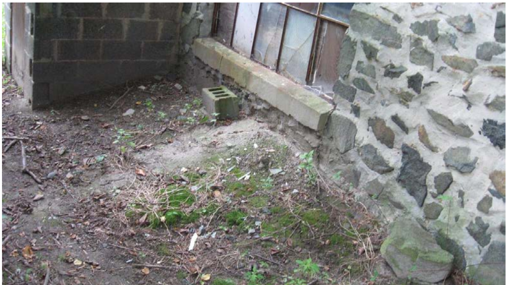
Powhatan Site – asbestos waste “dust” seeping out of building
