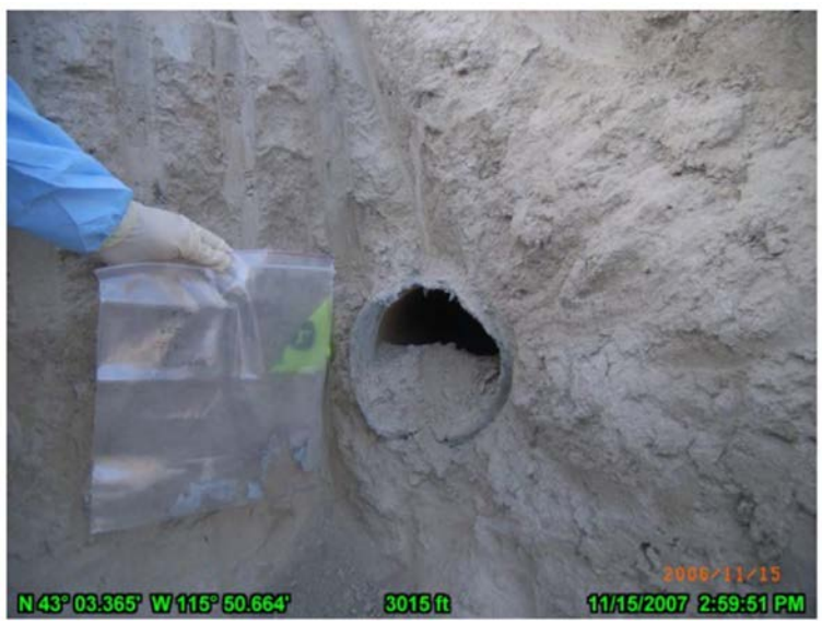
Mountain Home AFB – 2007 – Cement Asbestos Pipe (chrysotile and crocidolite)
