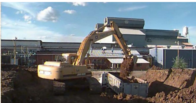
Clay donated by a local glass manufacturer to cap waste on site. (Source: ODEQ)
