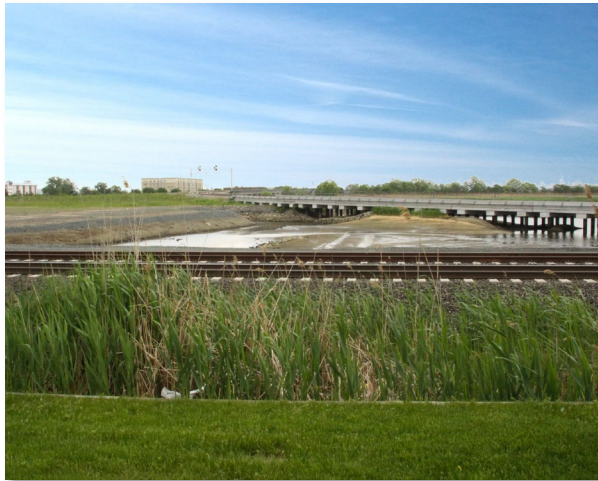
Figures 8-10. Rail line construction, April 2008 (Source: NJSEA). Rail line construction, December 2008 (Source: NJSEA). The Pascack Valley Line in the foreground and the Meadowlands Rail Spur in the background in 2013.
