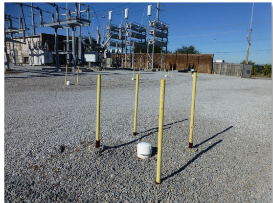
Figure 5. An extraction well at the SCE&G substation.
