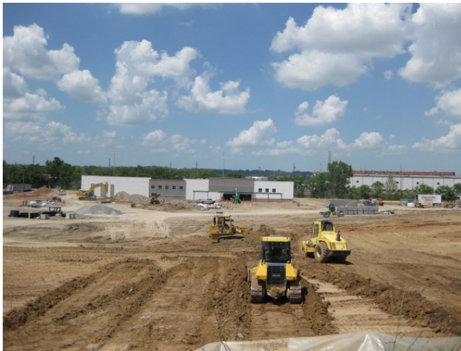
Kansas City Structural Steel removal site showing construction of retail space in 2014 following cleanup.
