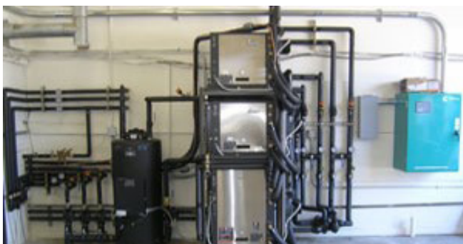
Figure 21. The geothermal heating and cooling system at the Arsenic Trioxide site.
