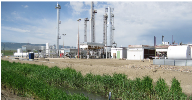
Figure 24. An active gas compression facility at the Mystery Bridge Road/U.S. Highway 20 site.
