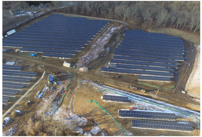
Figure 105. Aerial view of the solar facility at the West Kingston Town Dump/URI site solar farms (Rhode Island). Photo used with permission of Kearsarge Energy.
