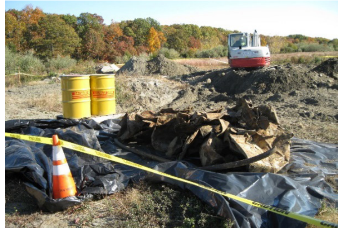
Figure 107. View of cleanup activities at the Davisville Naval Construction Battalion Center site (Rhode Island).
