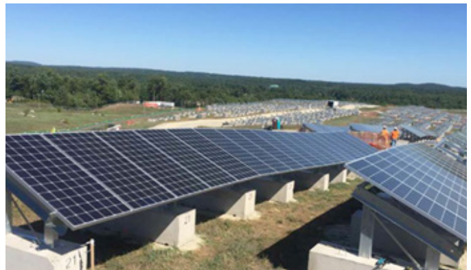
Figure 62. Solar panels at the Charles George Reclamation Trust Landfill site (Massachusetts).
