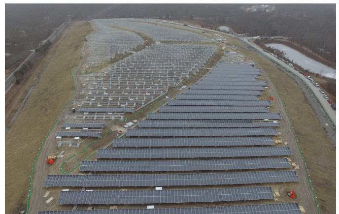
Figure 104. Aerial view of solar facility at the Rose Hill Regional Landfill site (Rhode Island). Photo used with permission of Kearsarge Energy.
