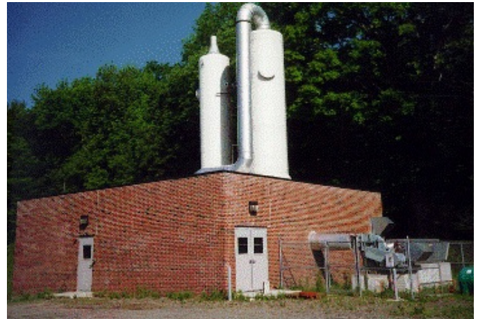
Figure 95. Facilities at the South Municipal Water Supply Well site (New Hampshire).
