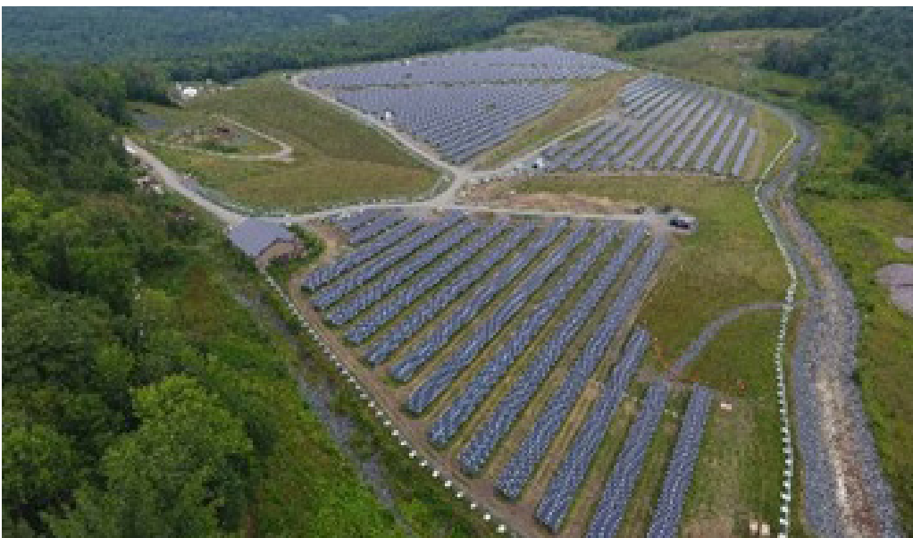
Figure 18. Aerial view of the solar array at the Elizabeth Mine site (Vermont). Image used with permission of Weston and Sampson, Conti Solar, and Elizabeth Mine Solar I, LLC.
