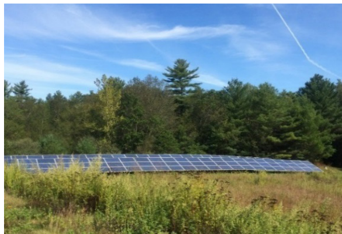
Figure 70. Solar panels at the Re-Solve, Inc. site (Massachusetts).
