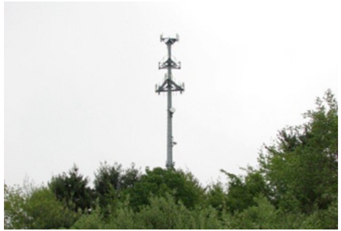
Figure 61. Cell phone tower at the CEC site (Massachusetts).
