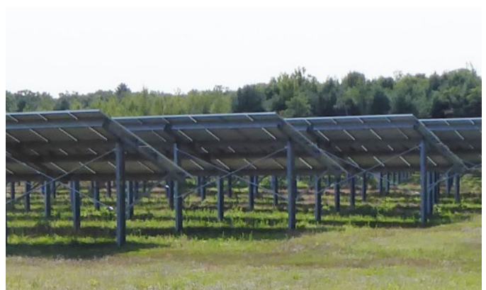
Figure 63. The solar facility at the Groveland Wells site (Massachusetts).
