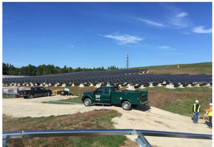
Figure 13. Installation of solar panels at the Charles-George Reclamation Trust Landfill site (Massachusetts).
