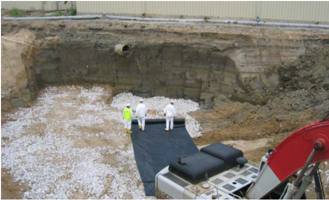
Phase 2 removal excavation up to the wall of the hardware store next to the site.
