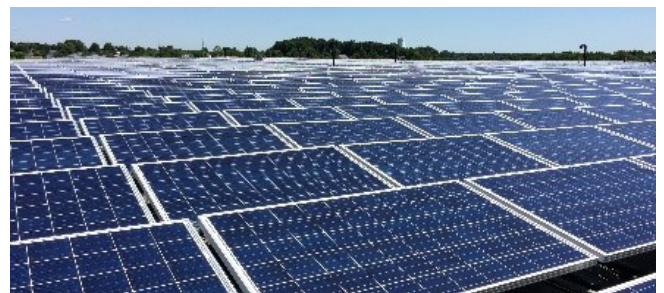
Figure 10. Solar array at the Brick Township Landfill site (New Jersey).
