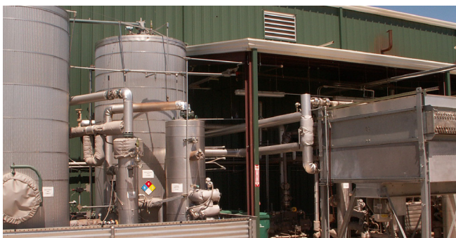
Figure 23. The award-winning gas-to-liquid fuel technology demonstration project.
