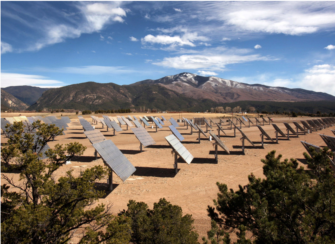
Figure 1. Solar facility at the Chevron Questa Mine site (New Mexico).
