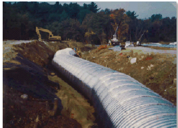
Figure 4. Installation of the Neponset River culvert prevents water from coming into contact with non-hazardous contamination in soil.
