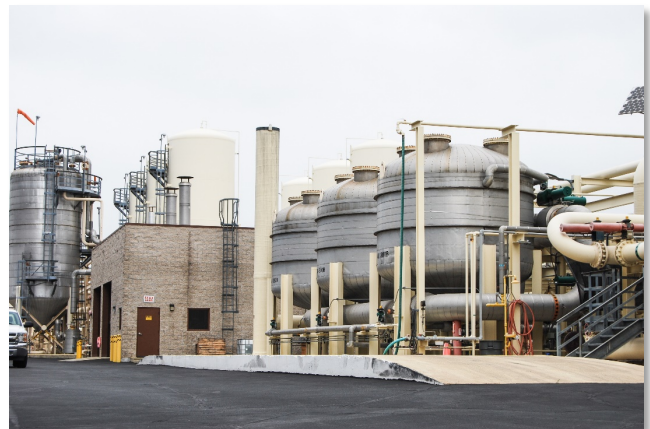
Figure 5. Burbank Water and Power water treatment plant. Image used with permission of Burbank Water and Power.
