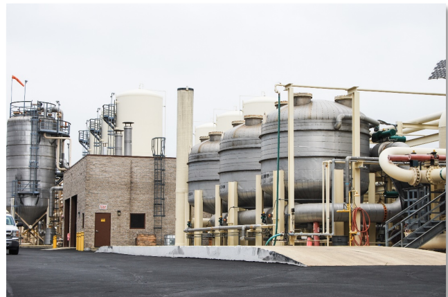
Figure 5. Burbank Water and Power water treatment plant. Image used with permission of Burbank Water and Power.
