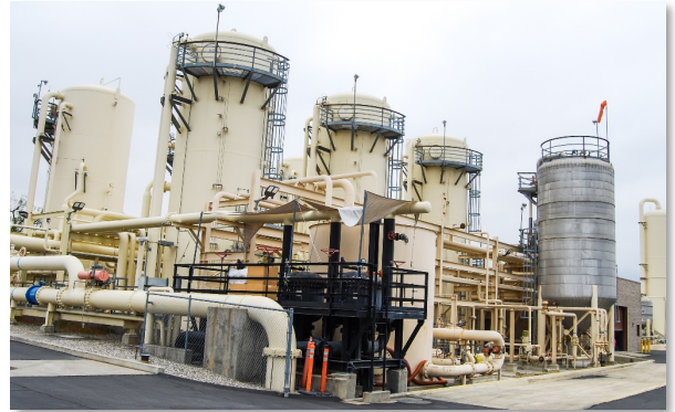
Figure 7. Burbank Water and Power water treatment plant. Image used with permission of Burbank Water and Power.
