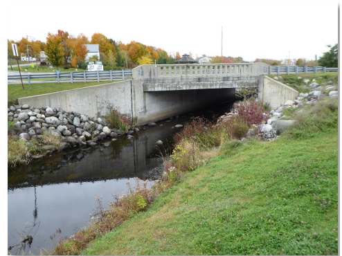
Figure 2. A view of the Route 7 bridge installed as part of the cleanup.
