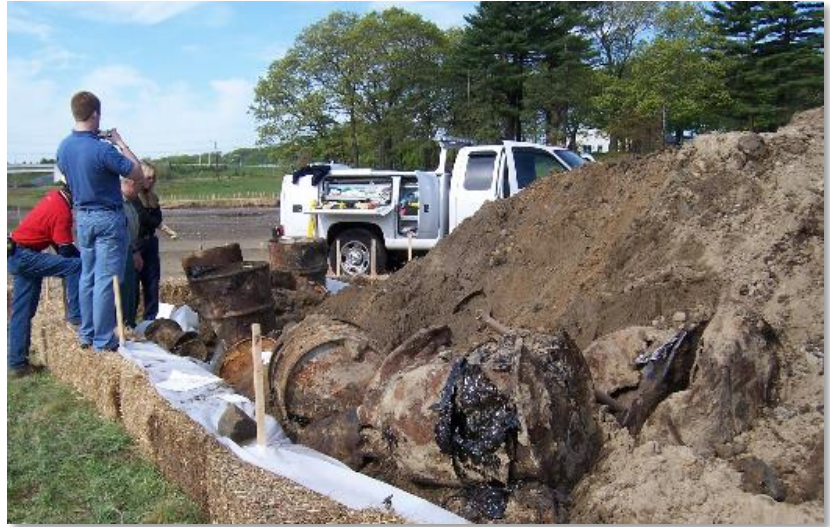
Figure 6. Cleanup efforts to address drums and contaminated soil on site. Image source: U.S. Navy.
