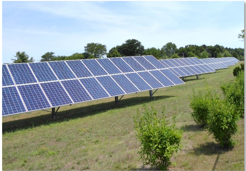
Figure 19. Ground-mounted solar installation along Davisville Road.
