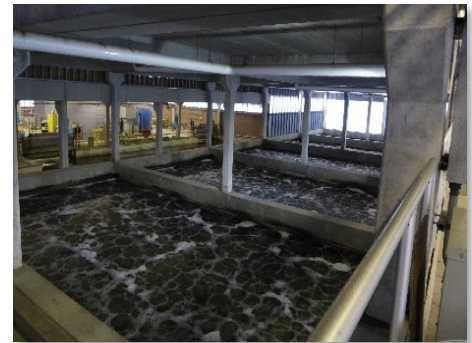
Figure 8. Metro state of the art facility and upgrades
