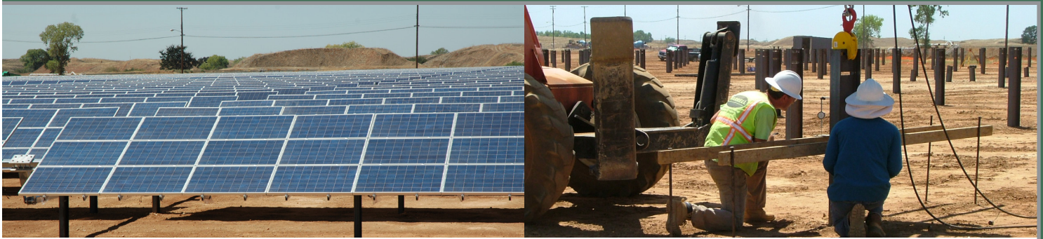
Images from left to right: On-the-ground view of facility solar panels and the facility under construction.
