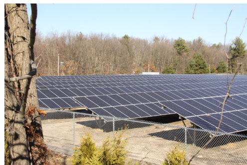
Figure 8. Completed solar panel array near the Iron Horse Park entrance.
