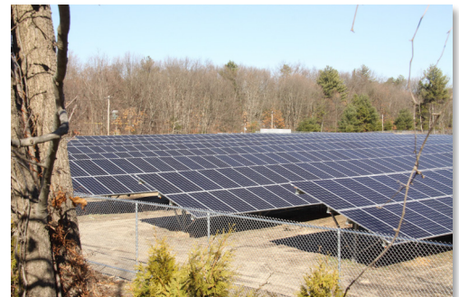
Figure 8. Completed solar panel array near the Iron Horse Park entrance.
