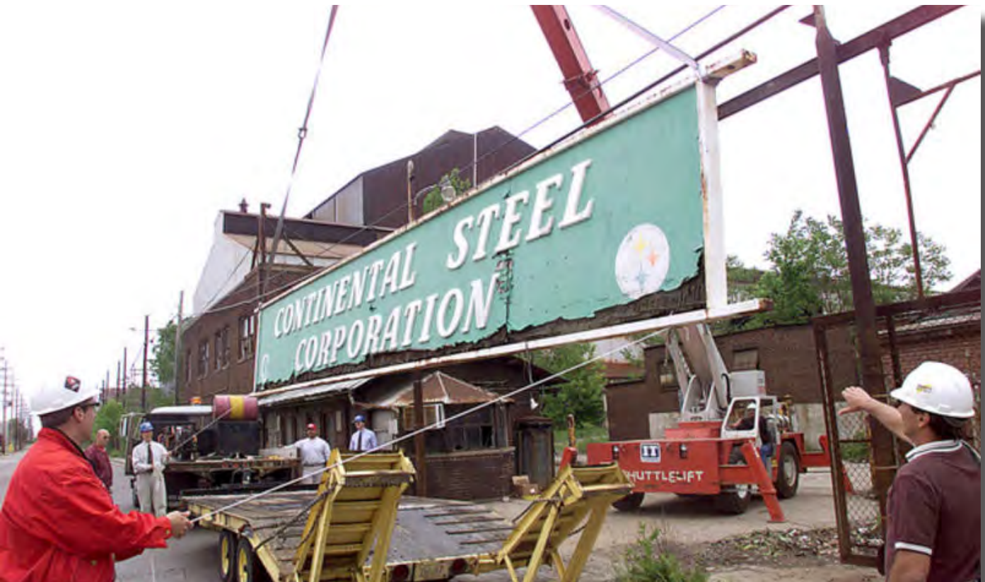
Company sign taken down in 1999, marking the beginning of building demolition efforts. (Source: Kokomo Tribune)
