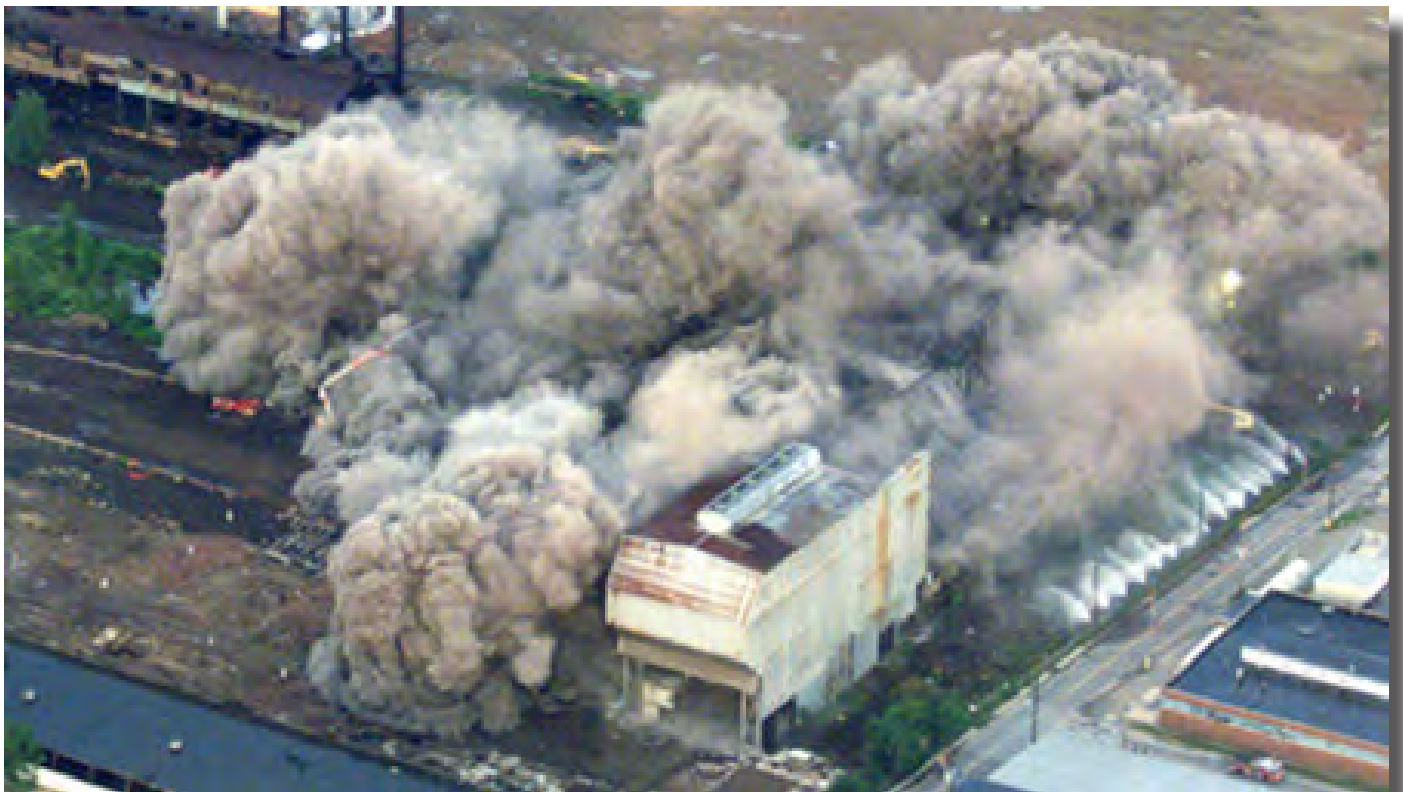
Demolition of the wire mill generated a huge cloud of dust. The wire mill was the largest building on site. (Source: IDEM)
