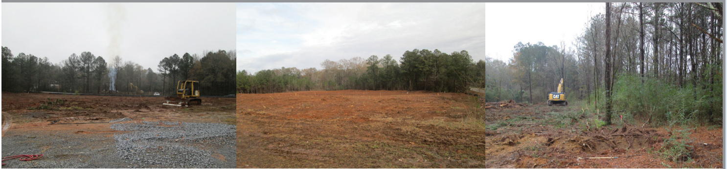
Images from left to right: View of the site cleared in preparation for groundwater injections, a cleared area of the site, and site clearing in progress.
