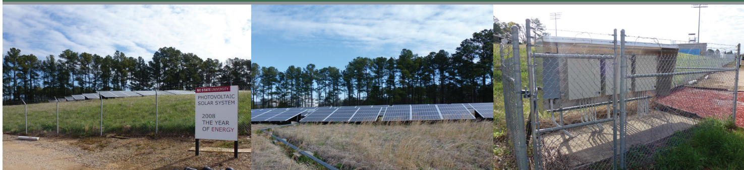
Images from left to right: Sign highlighting the photovoltaic solar system, solar panels on site and the solar panel control unit.
