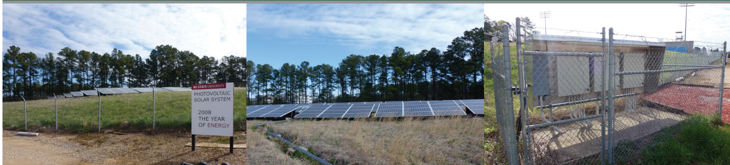
Images from left to right: Sign highlighting the photovoltaic solar system, solar panels on site and the solar panel control unit.
