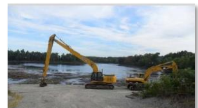
Figure 2. Dewatering activities associated with the former plow shop pond, as part of site cleanup.
