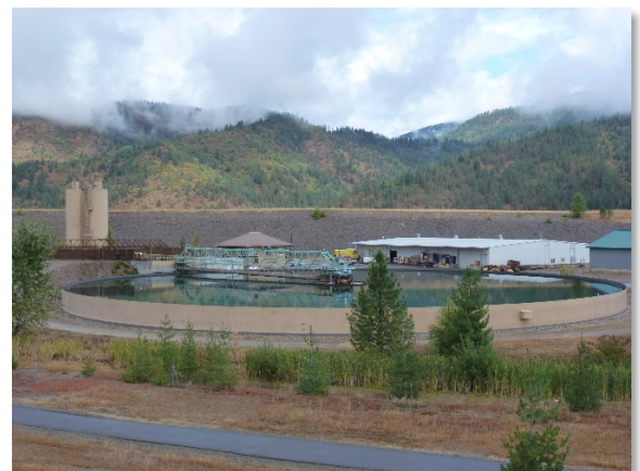
Figure 7. The site's Central Treatment Plant captures and treats mine drainage from the Bunker Hill Mine.
