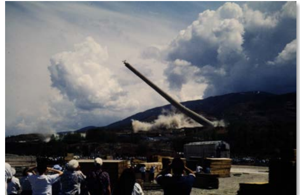
Figure 5. Demolition of the Bunker Hill lead smelter stack in 1996. Image source: Idaho PHD.
