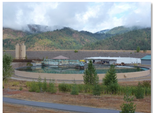
Figure 7. The site's Central Treatment Plant captures and treats mine drainage from the Bunker Hill Mine.
