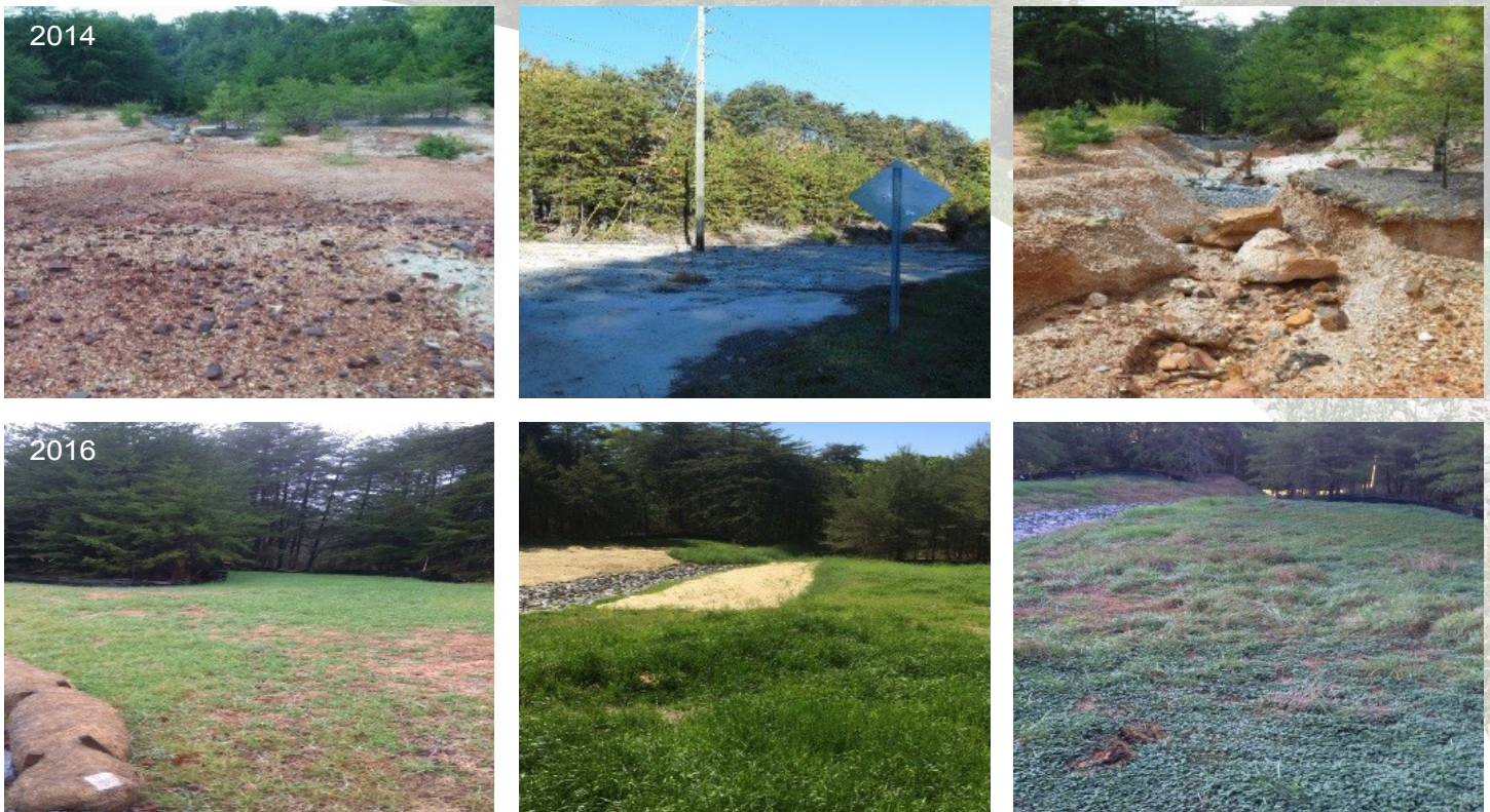
Figure 5. AOC 3 Vegetative Cover before construction (top row, 2014) and after construction (bottom row, 2016). (Source: ABB Inc.)
