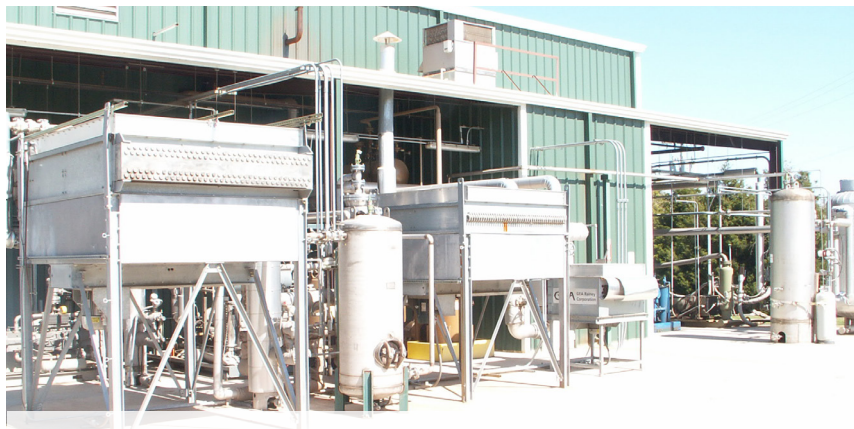
Figure 10: Methane gas-to-energy plant near the Mosley Road Sanitary Landfill site (Oklahoma)
