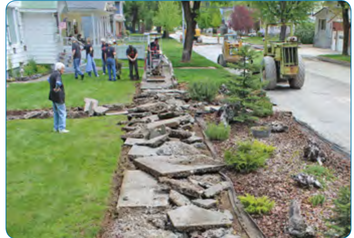
Volunteers planned to break up 129 feet of concrete and load it into wheelbarrows.
