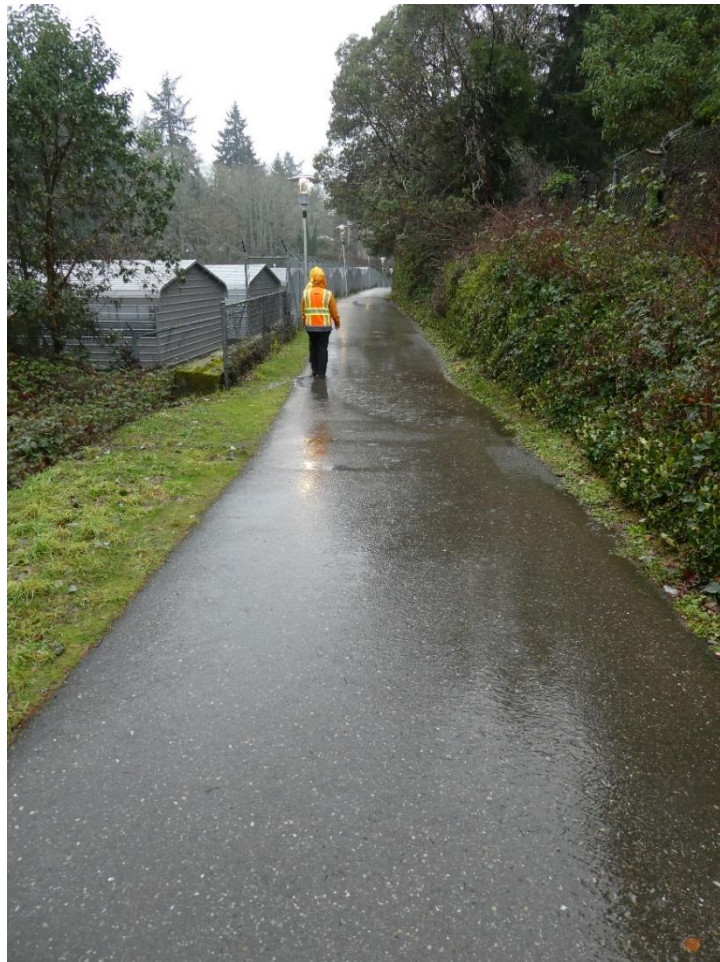
Ponded water near the northern drainage cutoff wall
