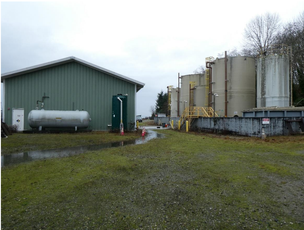
Groundwater treatment plant building and tank farm
