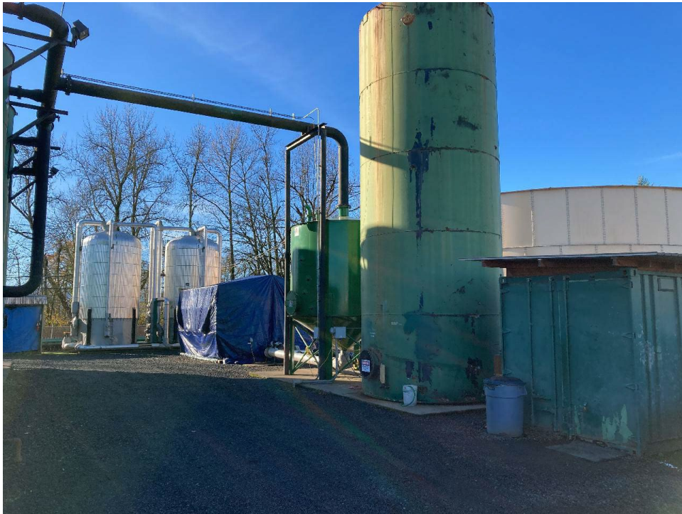
Stormwater and groundwater treatment system
