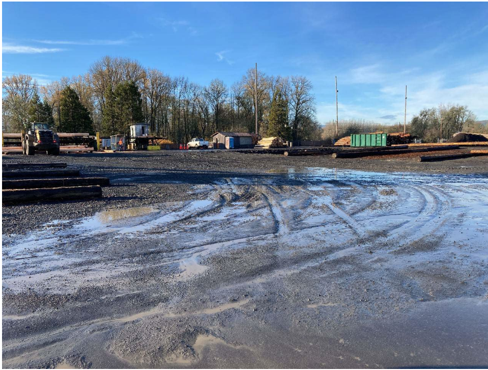
Minor ponding in the White Pole Storage Area
