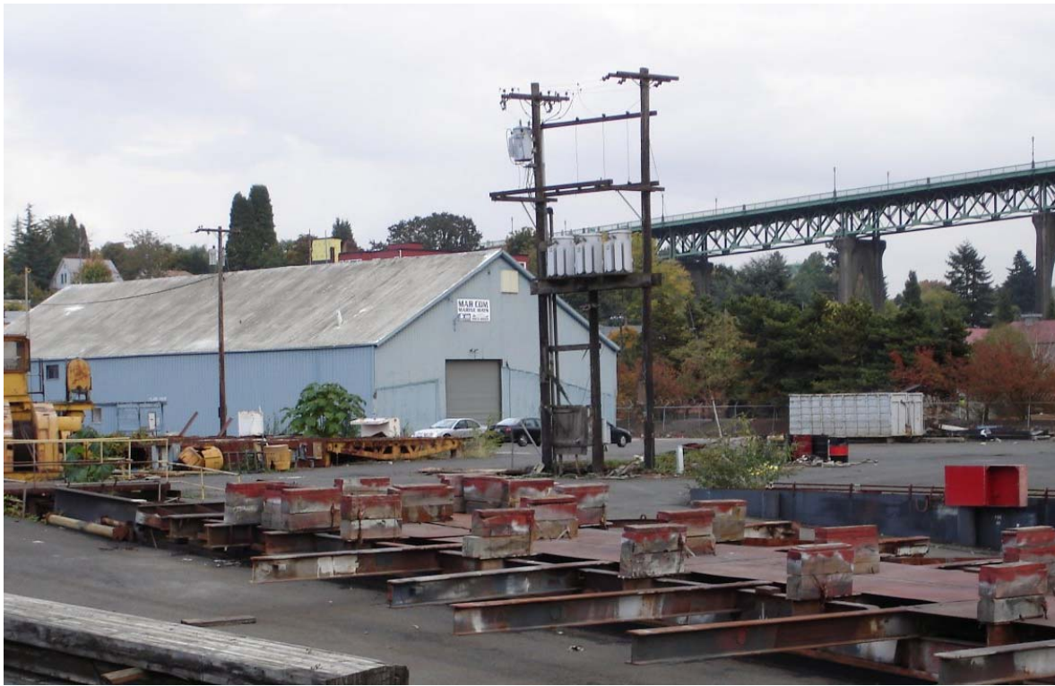
Photo 1: Site Photograph from June 2006 showing the three PGE transformers
