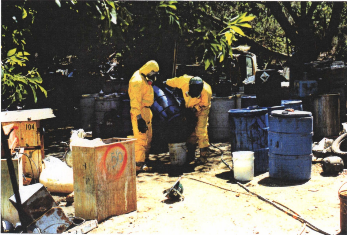
Drum decontamination; triple rinsing with soda ash/water solution. Photographer: R. Randall Date 4/24/90
