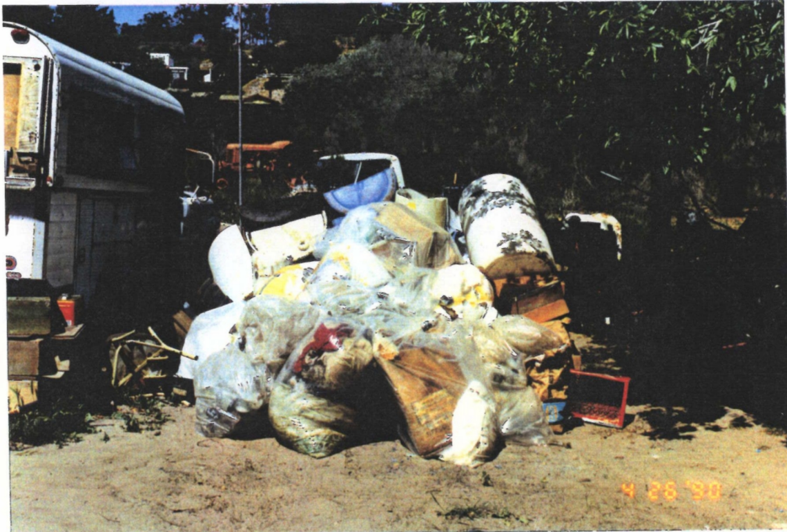
Removal generated debris and destroyed cyanide containers staged prior to placing in roll-off box for landfill disposal. Photographer: R. Randall Date: 4/26/90
