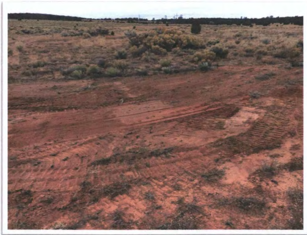
Photograph 14: View of typical removal of sharp metal feature with backfilling and compact on at Utility Raise U5 at Black Jack No. 1.
