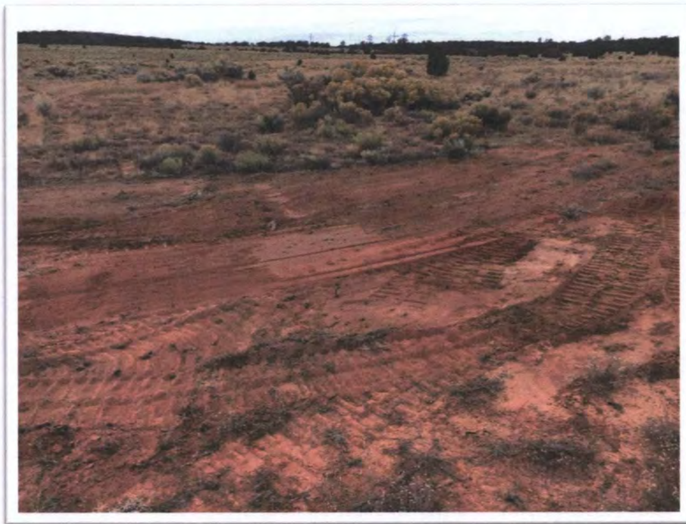
Photograph 24: View of typical backfilling, compaction, and grading of septic tank hazard at MAC No. 1.
