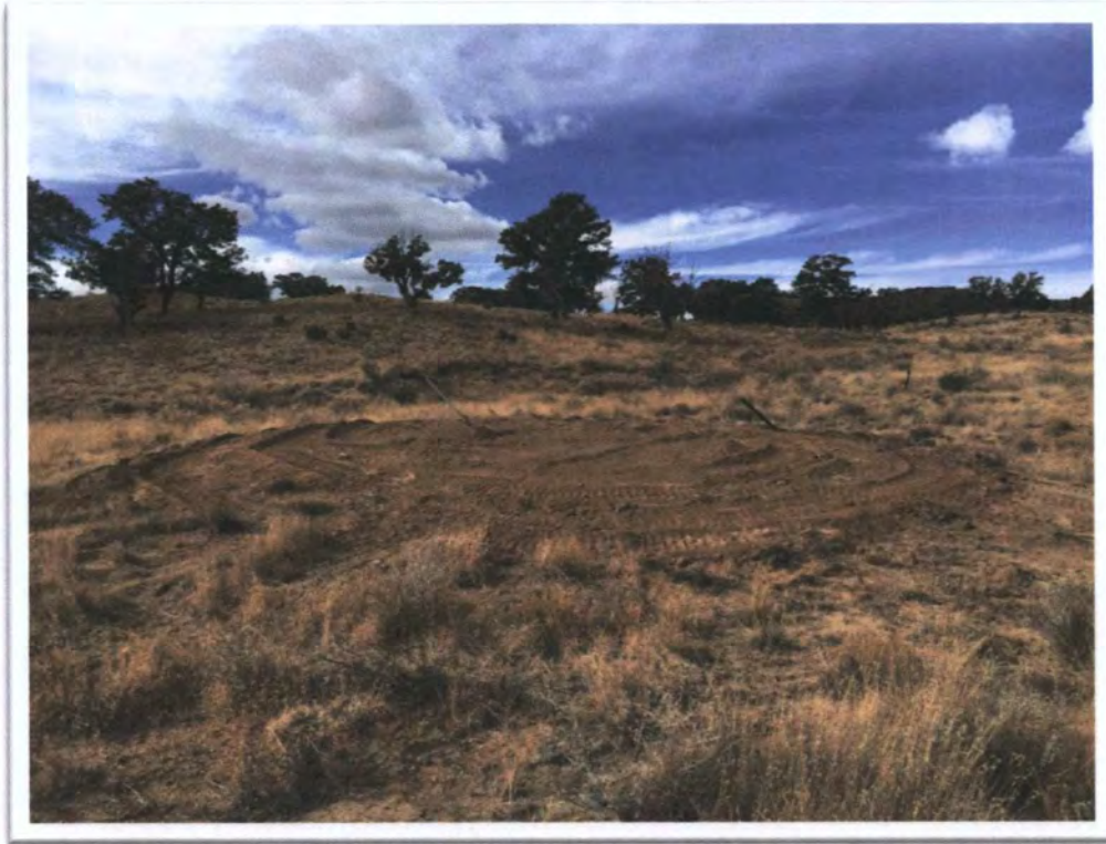
Photograph 11: View of typical backfilling, compaction, and grading at North Vent Shaft (NV) at Black Jack No. 1.
