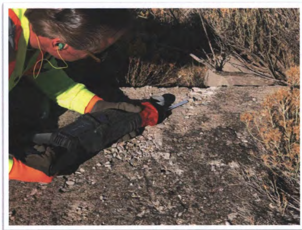
Photograph 4: View of typical cutting of wall anchor bolts flush with concrete slab at S2.
