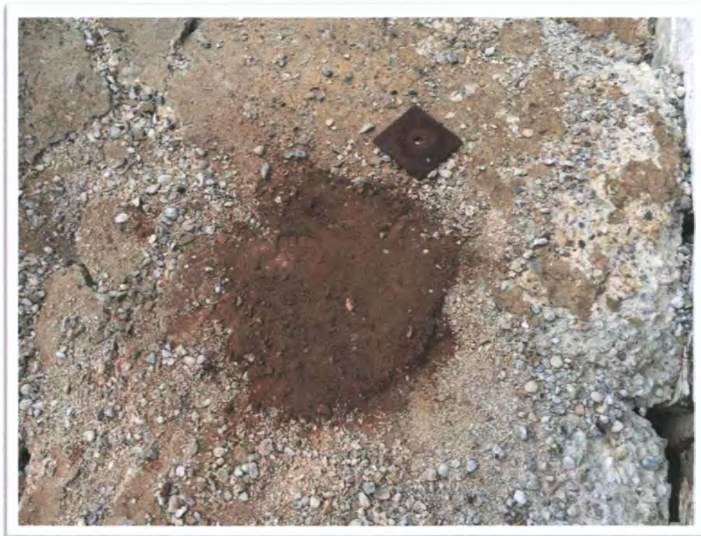
Photograph 22: View of typical cutting of sharp metal surface flush with concrete slab (S2) at MAC No. 1.
