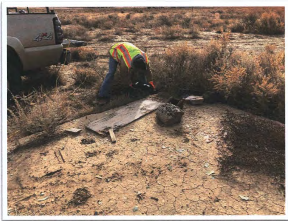
Photograph 3: View of typical cutting of wall anchor bolts flush with concrete slab at S1.
