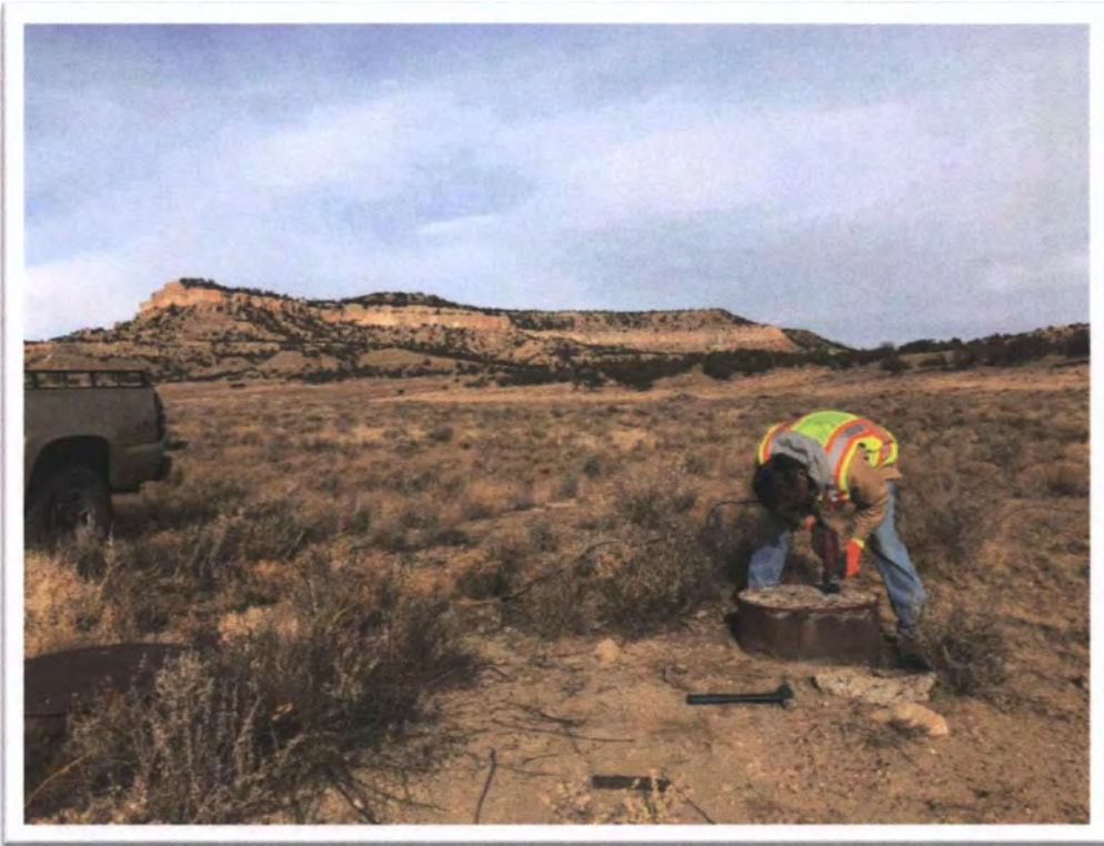
Photograph 9: View of typical cutting of hoist anchor bolts flush with concrete at central Vent Shaft at Black Jack No. 1.
