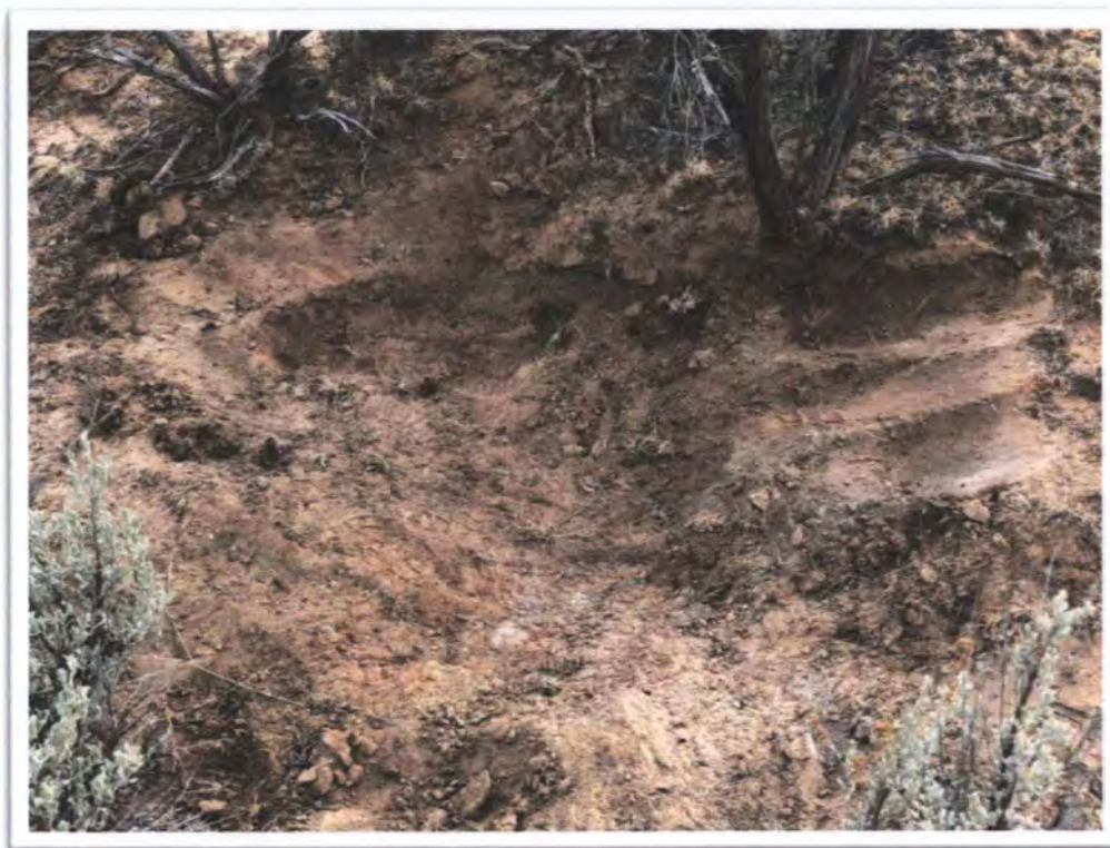
Photograph 28: View of typical backfilling, compaction, and grading at Vent Shaft-Borehole at MAC No. 2.
