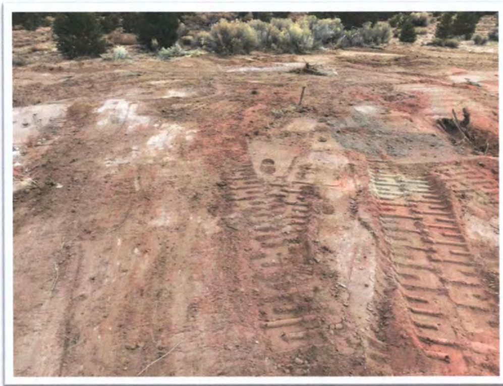
Photograph 19: View of typical backfilling, compaction, and grading of partially Buried Mine Shaft at MAC No. 1.
