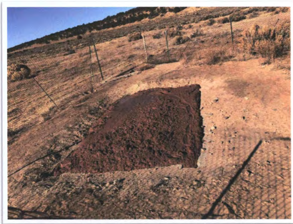
Photograph 15: View of typical flowable fill placement in Mine Shaft (MI) at Black Jack No. 2.
