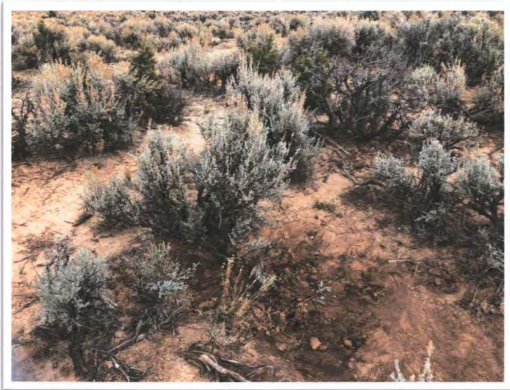
Photograph 26: View of typical backfilling, compaction, and grading of Open Hole (OH1) at MAC No. 2.
