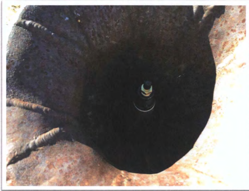
Photograph 13: View of typical inflatable packer (hole plug) installed in Utility Raise U4 at Black Jack No. 1.
