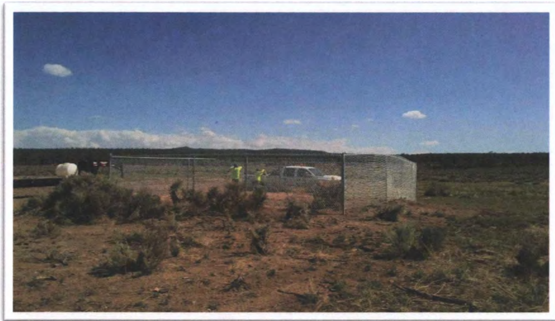
Photograph 29: View of new fencing installed around Mine Shaft (MK) at Black Jack No. 2.
