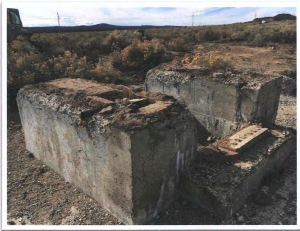
Photograph 6: View of typical Hoist House anchor bolts cut flush with concrete at Black Jack No. 1.
