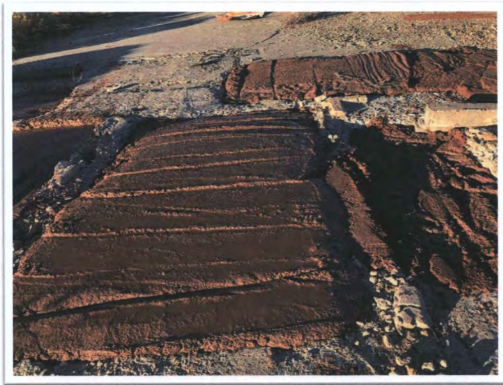
Photograph 7: View of typical placement of flowable fill into pits of Hoist House at Black Jack No. 1.
