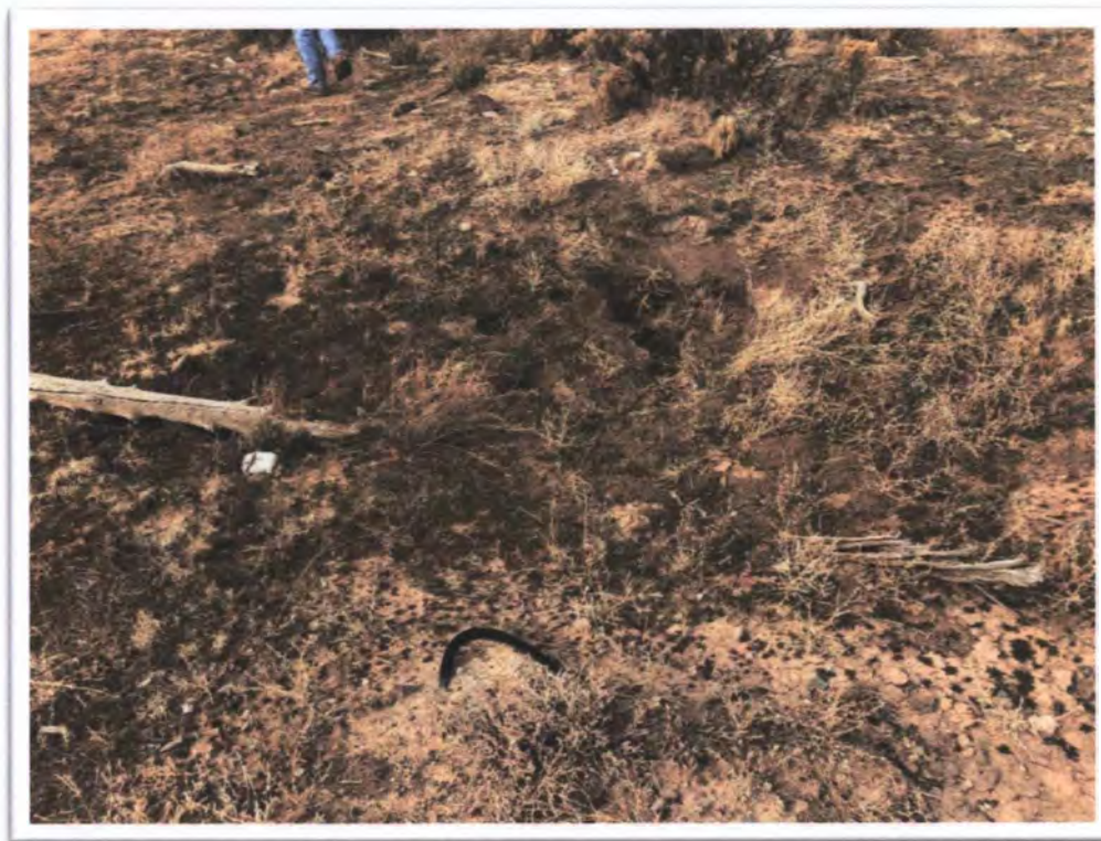
Photograph 16: View of typical backfilling and covering Utility Raise U1 at Black Jack No. 2
