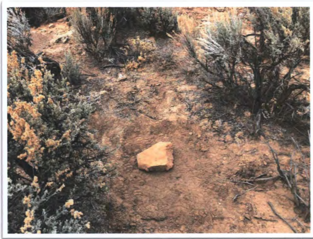
Photograph 27: View of typical backfilling, compaction, and grading at Open Hole (OH2) at MAC No. 2.
