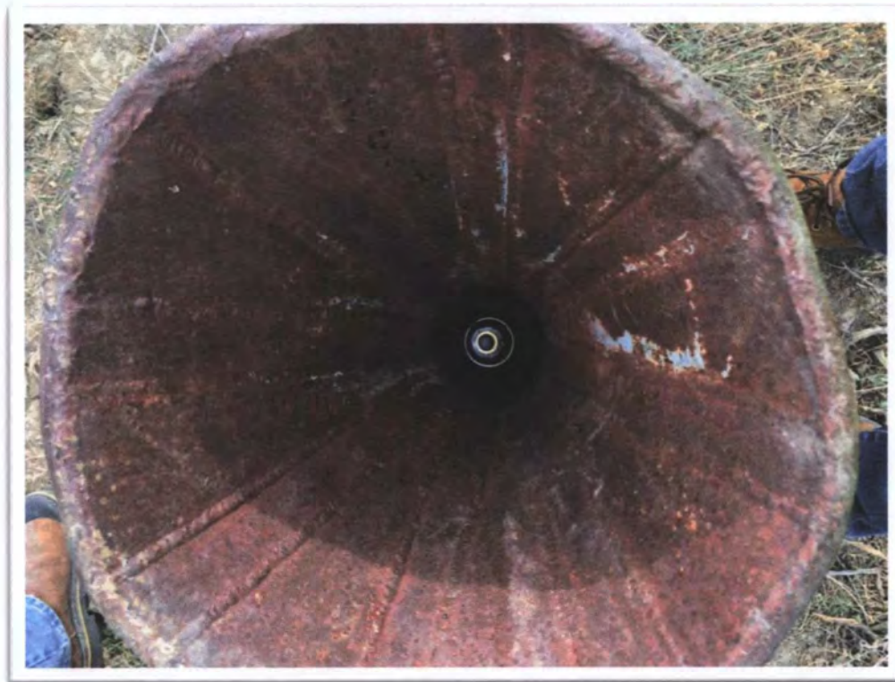
Photograph 12: View of typical inflatable hole plug installed in Open Hole (HS) and Utility Raise U4 at Black Jack No. 1.
