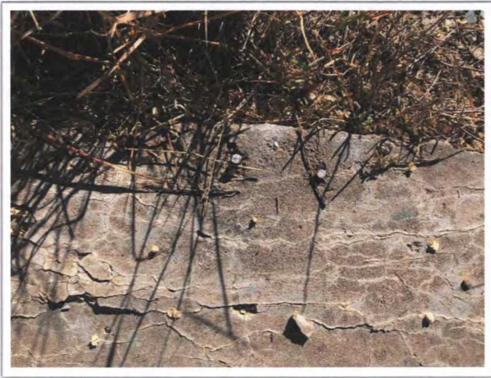
Photograph 5: View of typical wall anchor bolt cut flush with concrete slab at S3.
