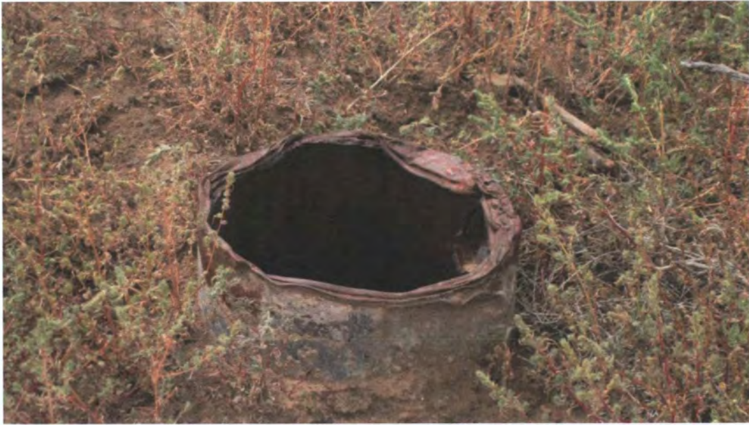
BJ2-7 Open south vent pipe west of main shaft
