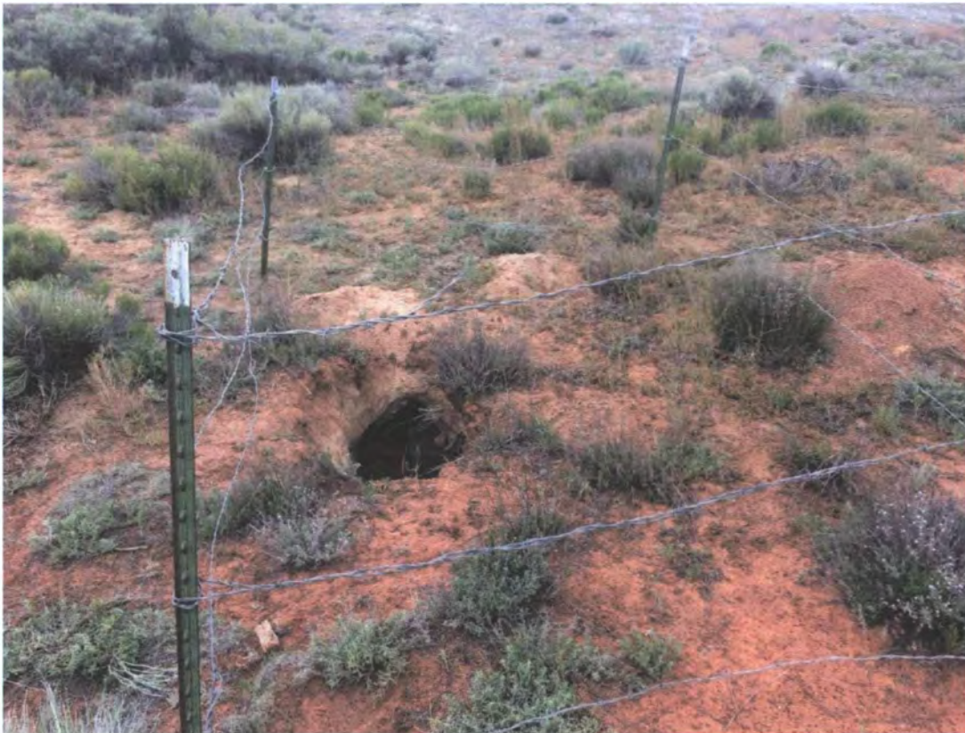
Mac 1-9 Uncovered vent raise south of office building with fencing installed in 2017
