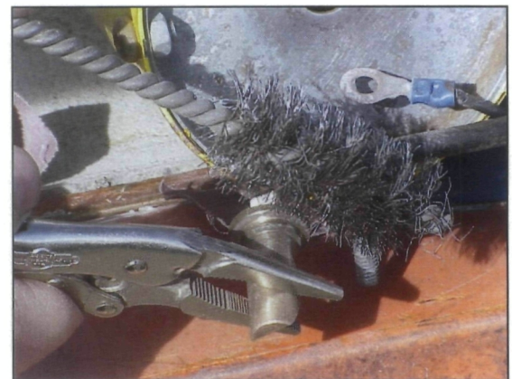
Figure 4. Corrosion on electrode. Use a wire brush, emery cloth or similar abrasive material to remove corrosion from point where electrode contacts the rear cover.
