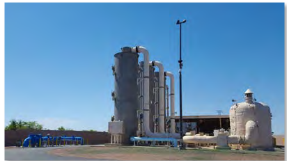
Figure 9. Air stripping towers at the TARP facility.
